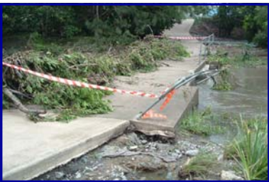
Turbulence underscores the causeway foundations and removes the vegetation.
